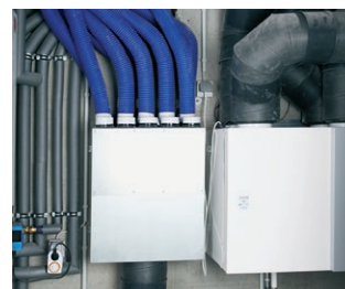
Insulated heating tubes
